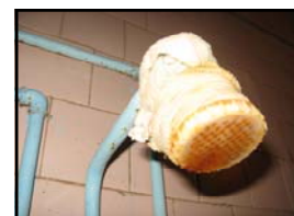
Inset: a dirty shower with only cold water.
